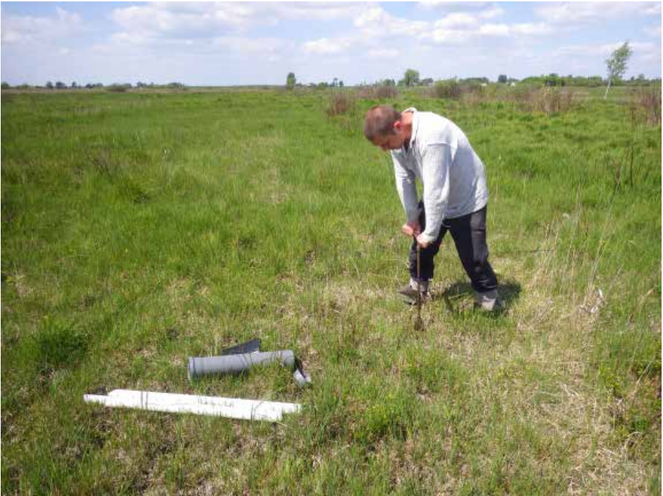
Photo 129: Installation of a piezometer with a measuring device (photo by E. Gutowska).
