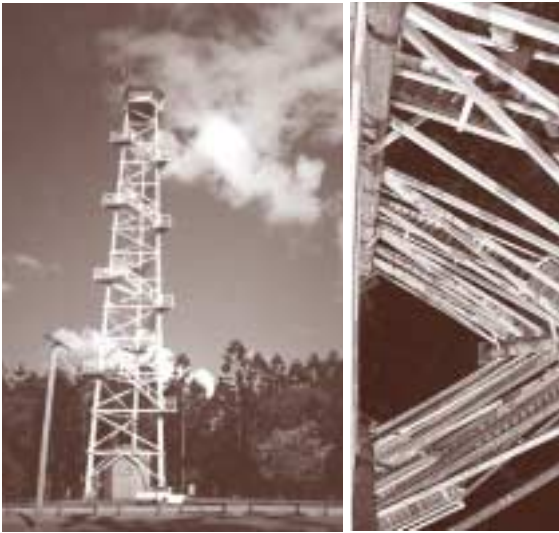
Queensland's tallest and opened in 1977, the 47-metre Jimna fire tower is listed on Queensland's Heritage Register but still plays a vital fire detection role. It is one of DPI Forestry's 49 fire towers.
