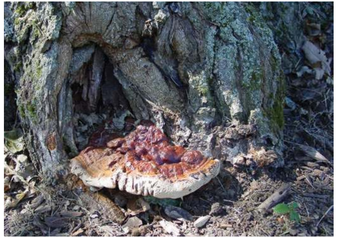
Photo 40. Mushrooms and conks indicate decay. Shown here: Ganoderma root and butt rot of bur oak. Also see Photo 88.
