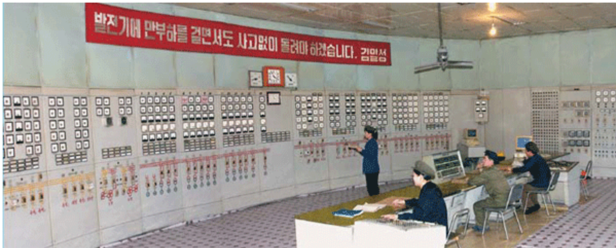
Figure 2-2: Control Room at Pukchang Thermal Power Plant 90
