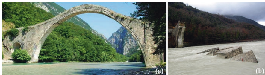
Fig. 5.10 Image of the Plaka Bridge before (a) and after (b) collapse
