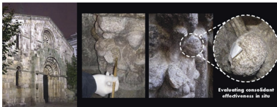
Fig. 12.3 Application and in situ evaluation of the UCA consolidants in the Church of Santa María del Campo (Galicia, Spain)
