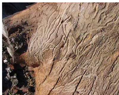
Figure 7.28. Larval galleries of the nautical borer ( Xylotrechus nauticus ). The granular frass was removed to show the pattern of the oval mines. Larval galleries appear to radiate outward from a common point. Like other wood-boring beetles, the eggs are deposited on the bark surface, not under it as with bark beetles. B. HAGEN
