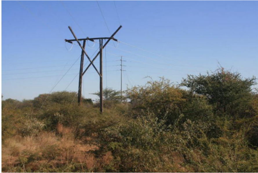
Figure 3. Lack of a track beneath the line makes passage difficult throughout.
