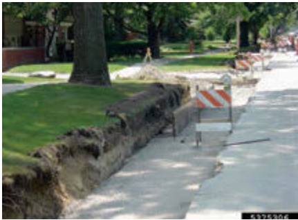
Fig. 10.6.11. Root damage caused by digging and trenching during sidewalk construction. USA, AKo.
