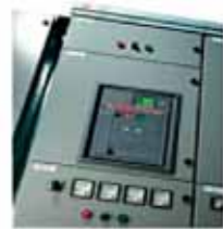
Faults: no problem
