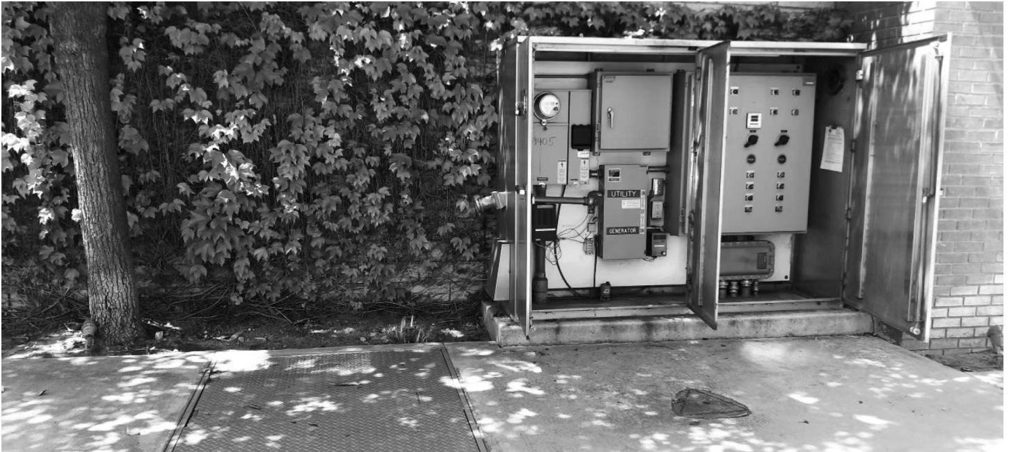
Carmenita Sewer Lift Station
