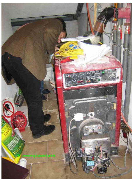
Oil boiler in Austria. Photograph:
