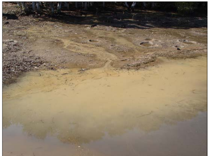
Sediment entering a waterway from a building site. (Source: Peter Adderley, 2003)
