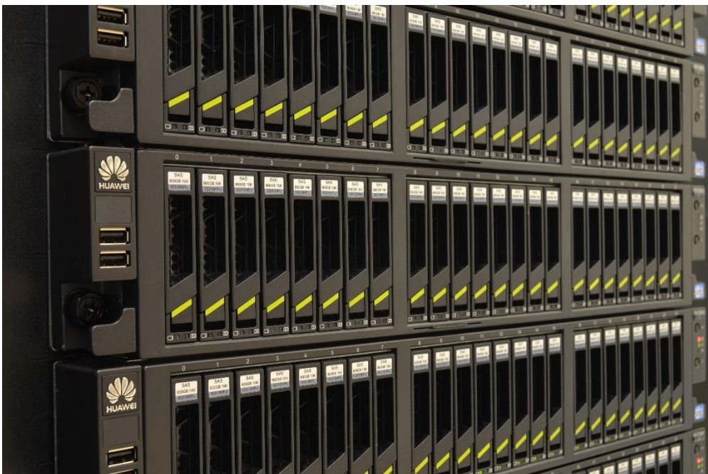
Storage servers with 24 hard disk drives and built-in hardware RAID controllers supporting various RAID levels
