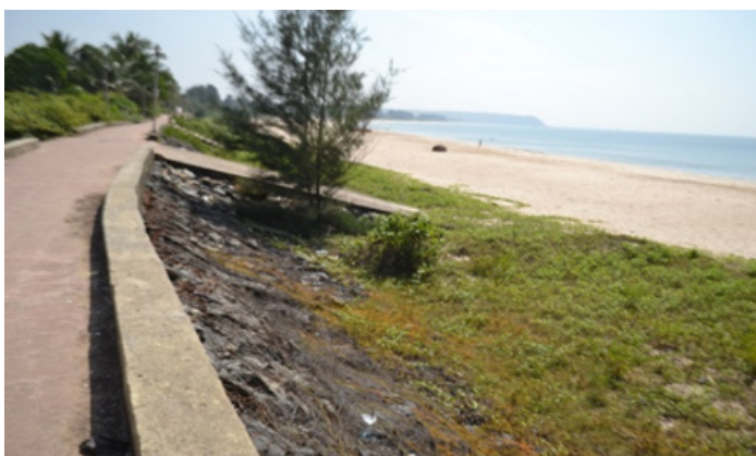
Revetment, vegetation and wide beach at Navabag, Vengurla, Sindhudurg, Maharashtra facilitating flood protection, fishing operations, recreation and tourism
