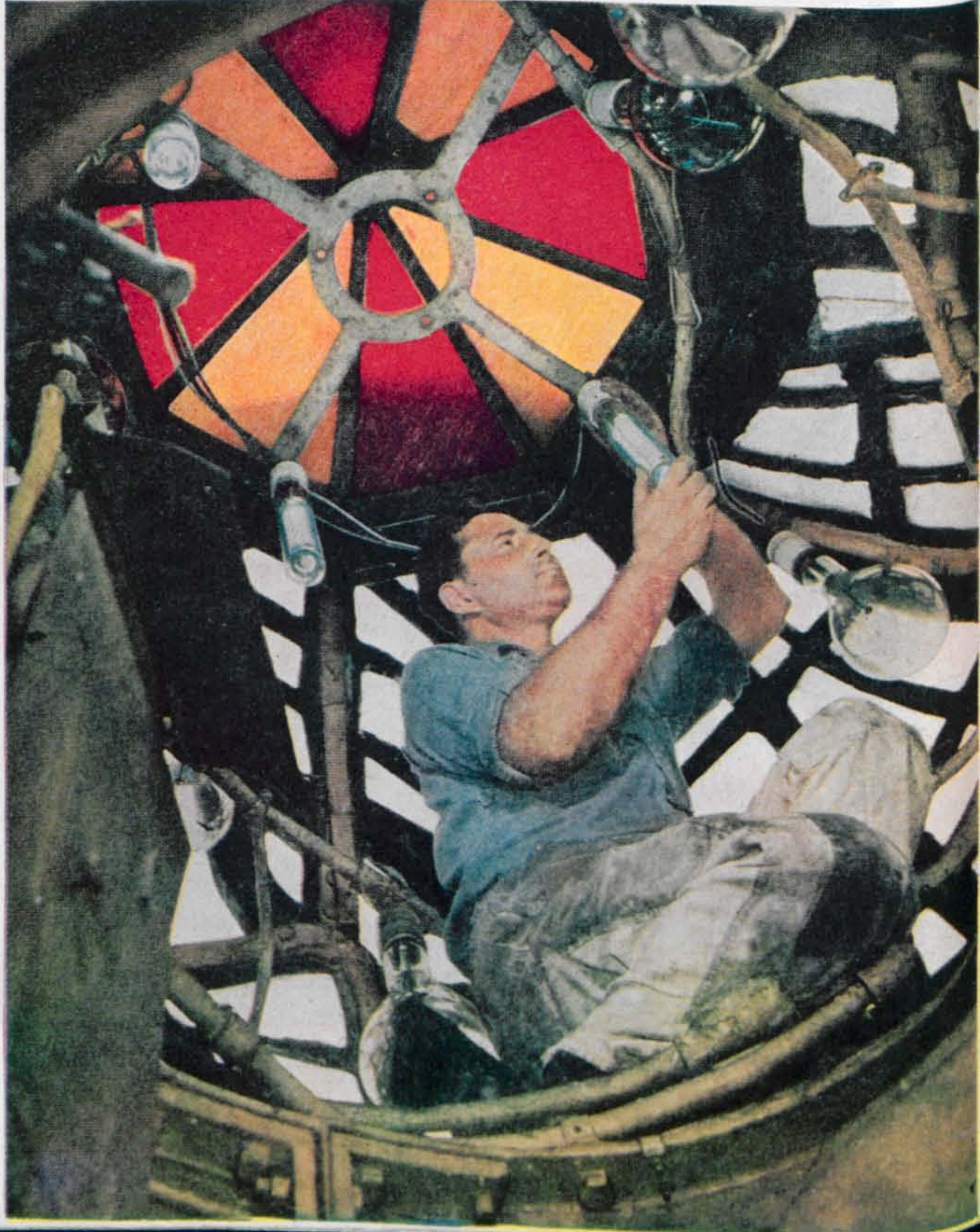
Lighted by a system of incandescent and mercury vapor lamps, the torch is a beacon to approaching ships. Here a workman replaces wind-smashed bulb.
