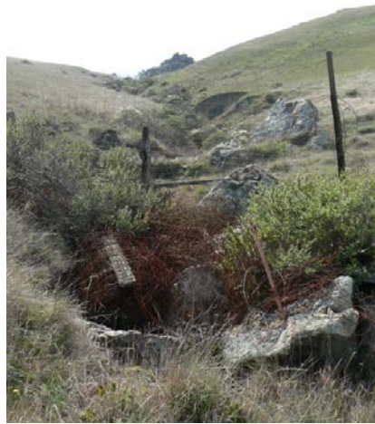
Photopoint 6. Gully 1 at property line
