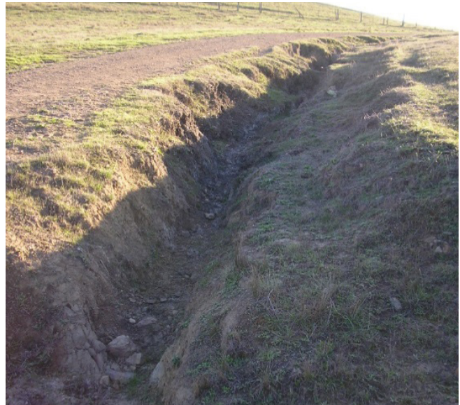
Erosion along Wright Hill Road
