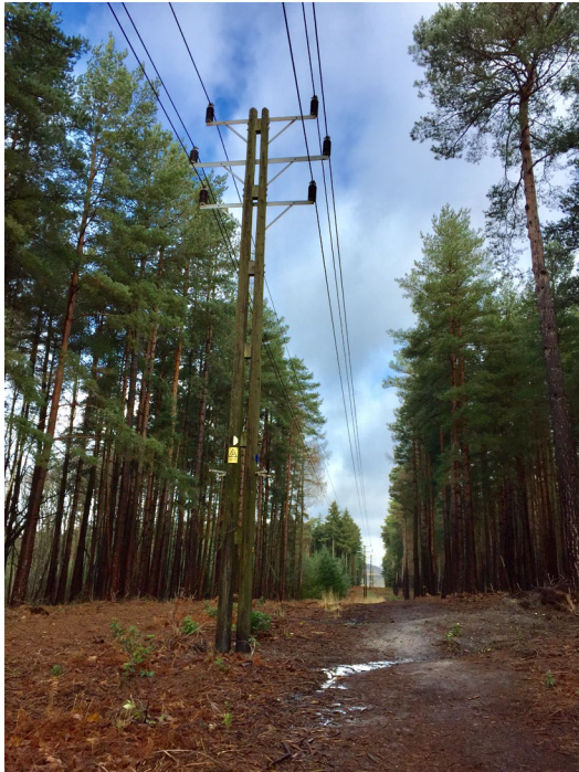
33kV power line
