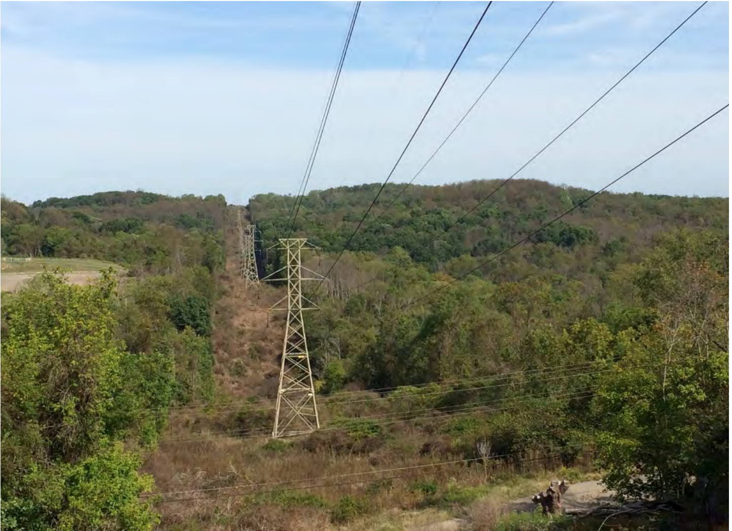
Power line running through Boyce Park.
