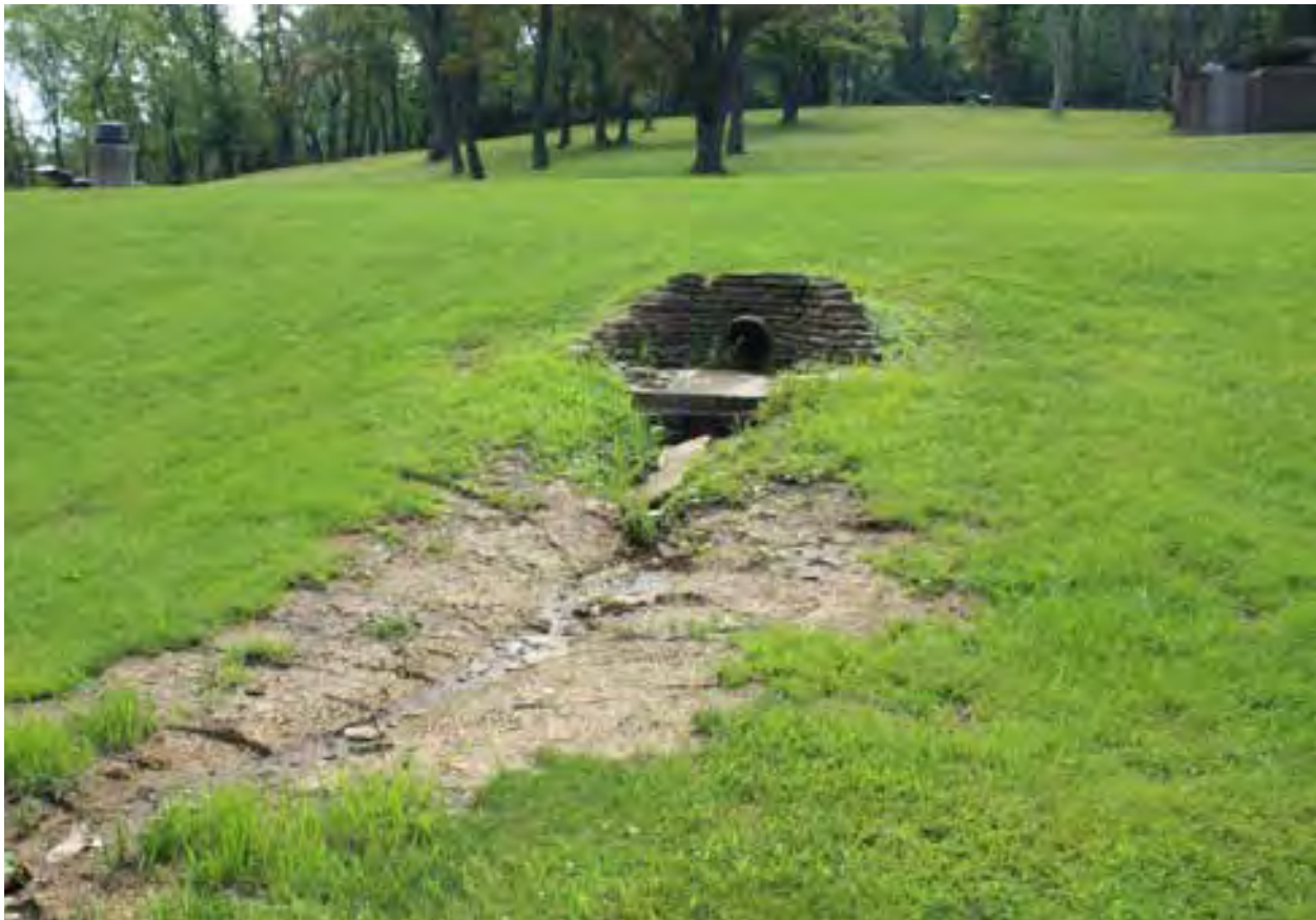
EU 69 - Erosion issues from roadway.
