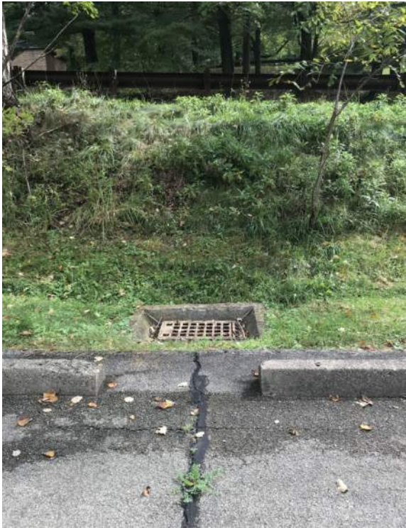
Catch Basin next to the Cedar Grove Lot.
