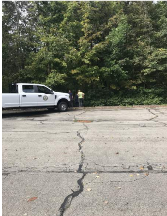
Catch Basin in the Center of Cedar Grove Lot, just above the Outfall Pipe
