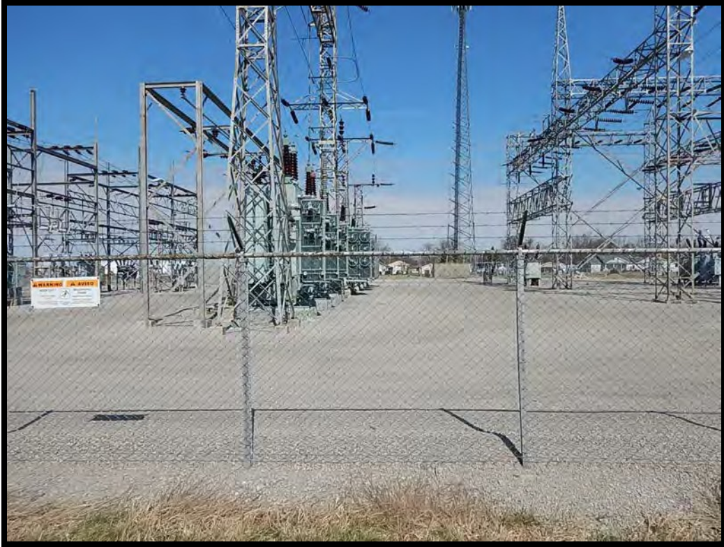
Figure 6. The existing substation within the western portion of the project.
