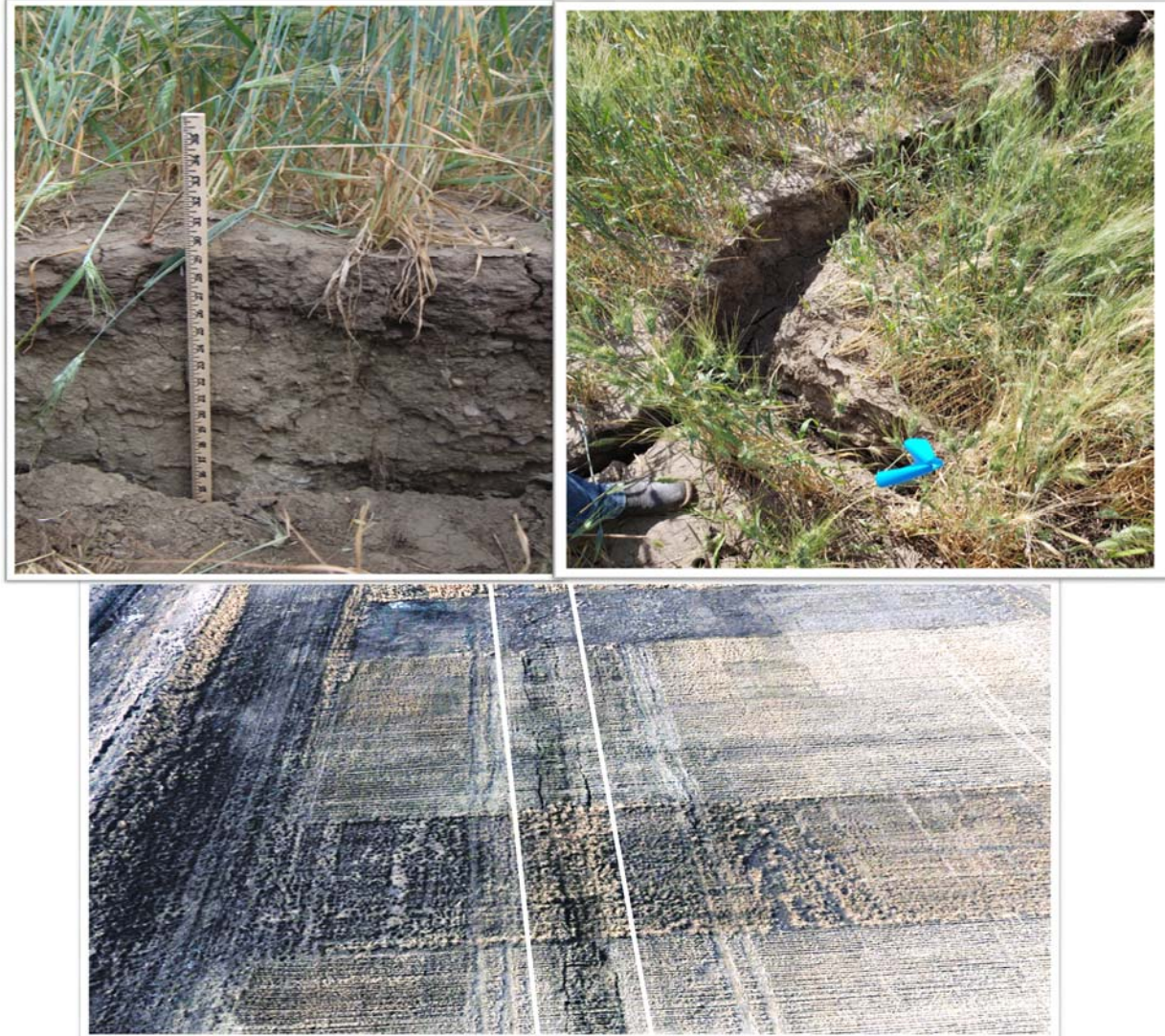
Figure 5. Images of subsidence along the pipeline disturbance area. The upper two images were taken shortly after the subsidence occurred in July 2018. The aerial image was taken in March of 2019, the sunken area is outlined in white.
