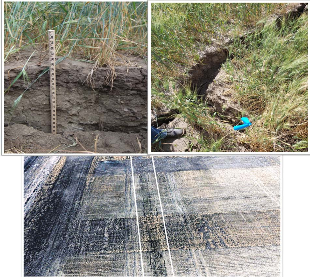
Figure 5. Images of subsidence along the pipeline disturbance area. The upper two images were taken shortly after the subsidence occurred in July 2018. The aerial image was taken in March of 2019, the sunken area is outlined in white.
