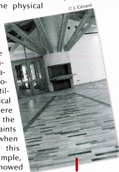
Parquet floor in holm oak, made for the CRPF.
