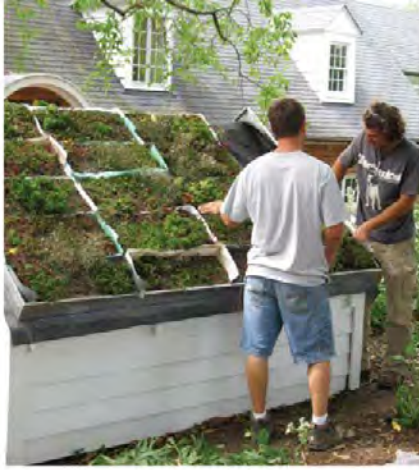
Crew members from Furbish install a green roof on the well house at River Farm.
