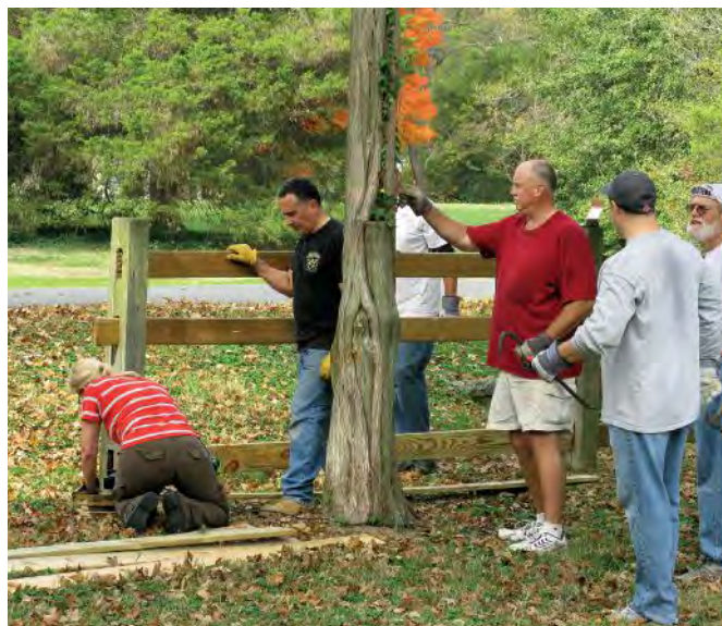
A group of SAP AG volunteers repair a fence at River Farm.
