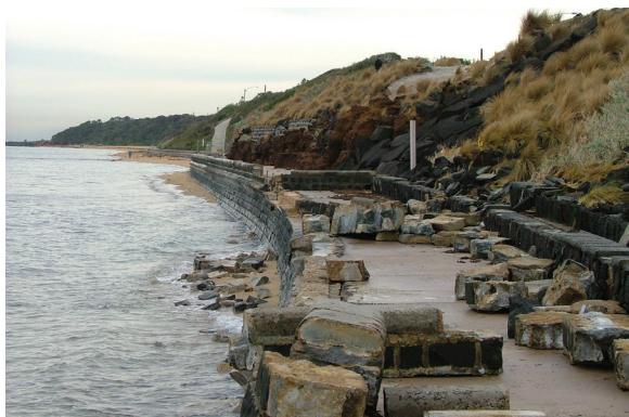
Figure 6.2 Significant storm damage to the Black Rock historic bluestone masonry seawall and promenade constructed in the 1930s is costly for land managers to repair (Photo: M Mitchell)
