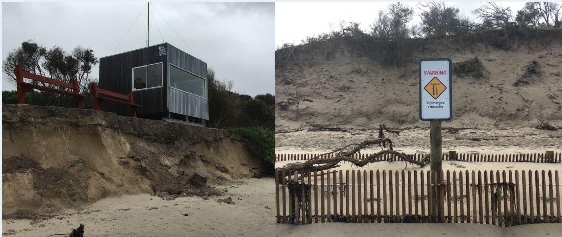
Left: Erosion undermining the Inverloch patrol tower in 2018 has continued. Right: Wet sand fence after completion in early 2019 (Photos: A Kilborn)
