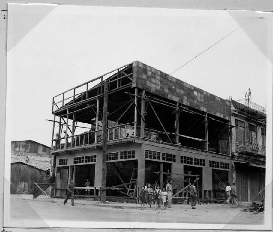
This building is typical of the flimsy, knocked-together sort of building which is going up in the Manila business district today. There is no steel, no concrete, no lumber, no glass in sufficient quantity to replace the great stone buildings that lined Juan Luna and the Escolta in pre-war Manila.
