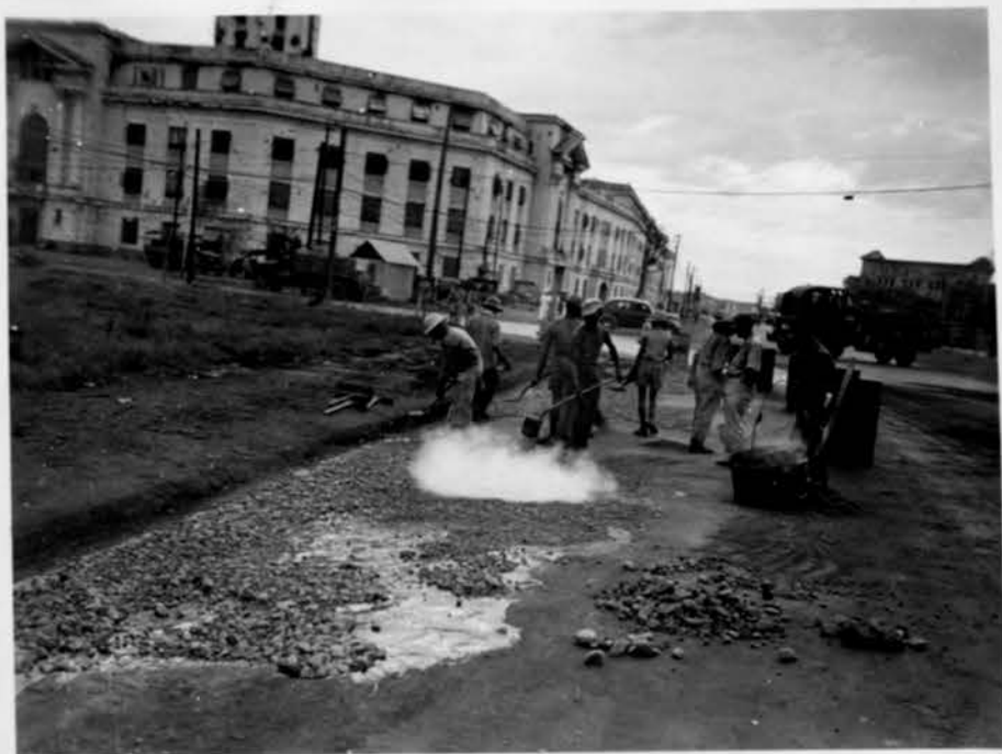
Repairing the streets of Manila is an endless job because of the scarcity of material and heavy equipment.
