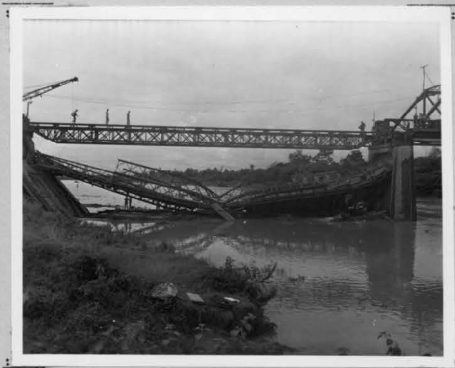
This bridge is part of the National Highway system and crosses the Mariquina River. Its repair was undertaken to serve the Army depots in the Mariquina River district.
