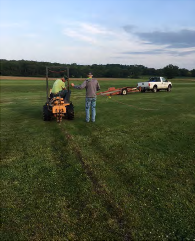
Carl Dowse, Site One Irrigation and Justin Johnson from Olson-Toon Landscape install new irrigation wires.
