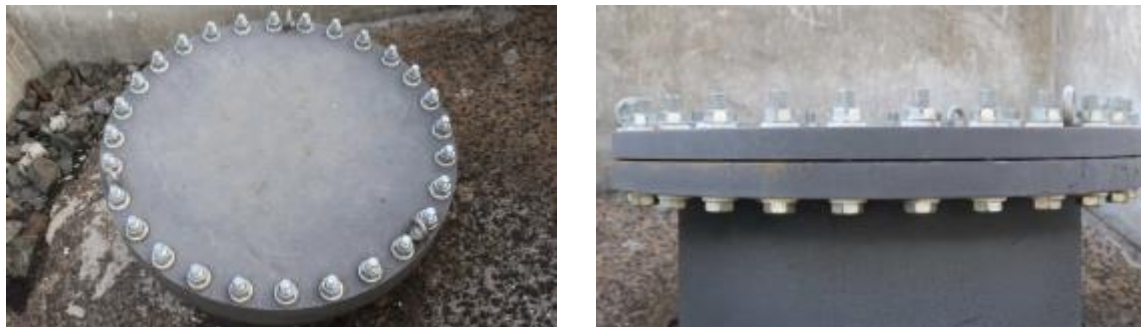
Figure 3-2: Connection to the existing flanges at Mt Coffee HPP.
