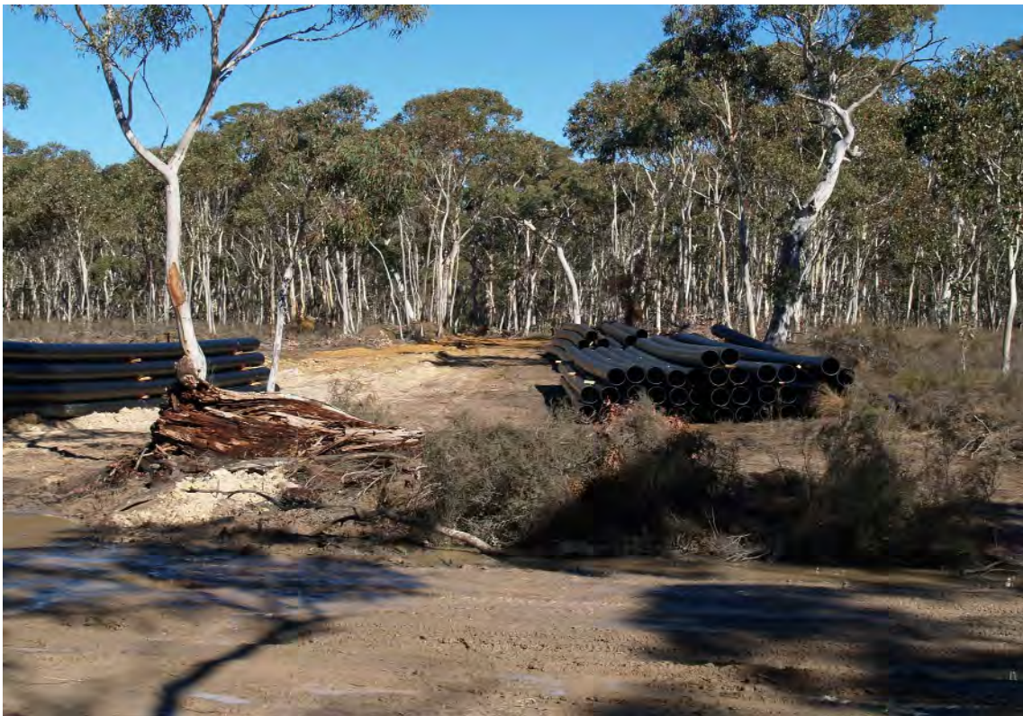
A nationally endangered shrub swamp was cleared and used for road construction and as a temporary pipe storage area, July 2005
