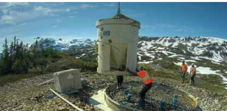
All told, about 20 million pounds of concrete will be moved to construct the foundations for the transmission towers. Bryan Dudas Photos
