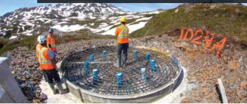
A tower foundation construction crew member stands on top of a rebar cage that will be filled with concrete flown in by an Airplane. This will then be topped with a 16,000-pound steel cap to complete the foundation.
