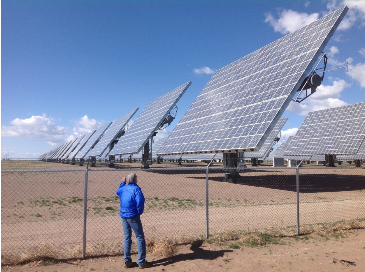
Figure 5.5-1. Close-Up View of Amonix 7700 CPV Panels at Alamosa Solar Generating Plant.
