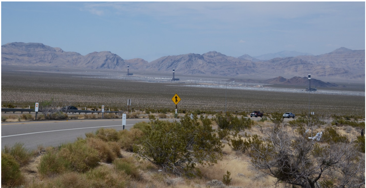
Figure 5.3–3. Ivanpah Power Tower Facility Under Construction from a Distance of 4.3 mi (6.8 km) from the Closest Tower, May 2013.
