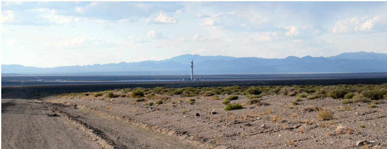
Figure 5.4–3. Crescent Dunes Solar Energy Project under Construction, as Seen from a Distance of Approximately 7.1 mi (11.4 km), May 2013.
