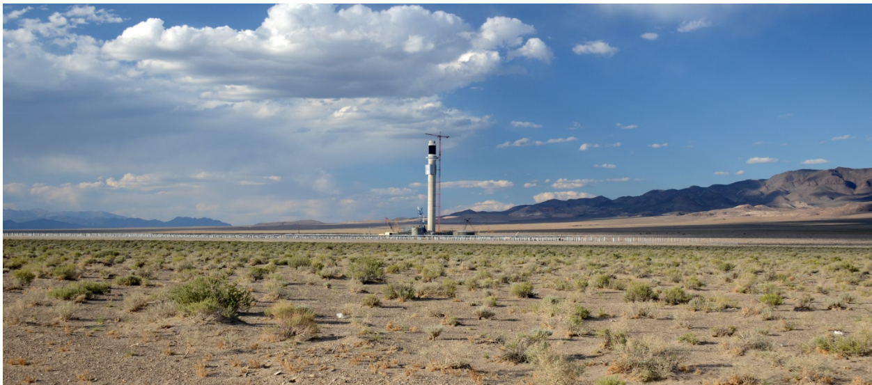
Figure 5.4–1. Crescent Dunes Solar Energy Project under Construction, as Seen from a Distance of Approximately 1.3 mi (2.1 km), May 2013.
