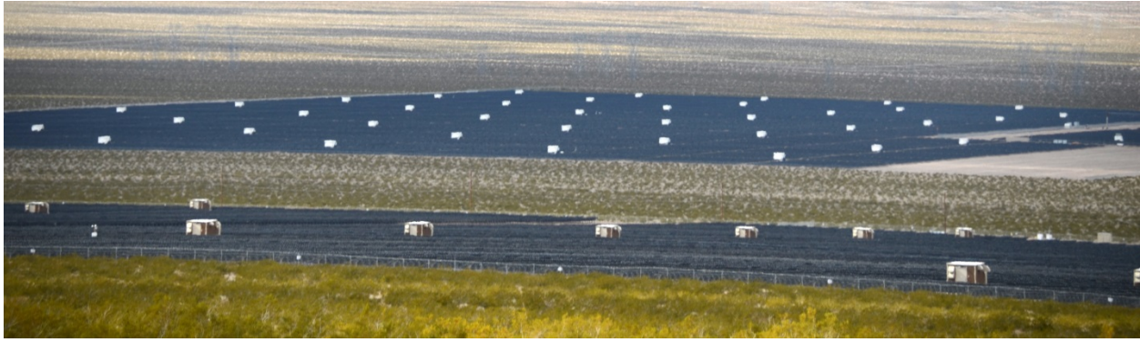
Figure 6.2–3. Brown/White PCUs at CM 2 Facility (foreground), White PCUs at CM 1 Facility (background).
