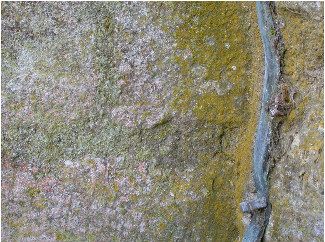
Caloplaca aff. austroclitina (deep golden yellow) growing as a metallophyte beside a lightning conductor (Riseley church, Bedfordshire). C. limonia (very pale yellow) is dominant on uncontaminated mortar courses in left half of the image.
