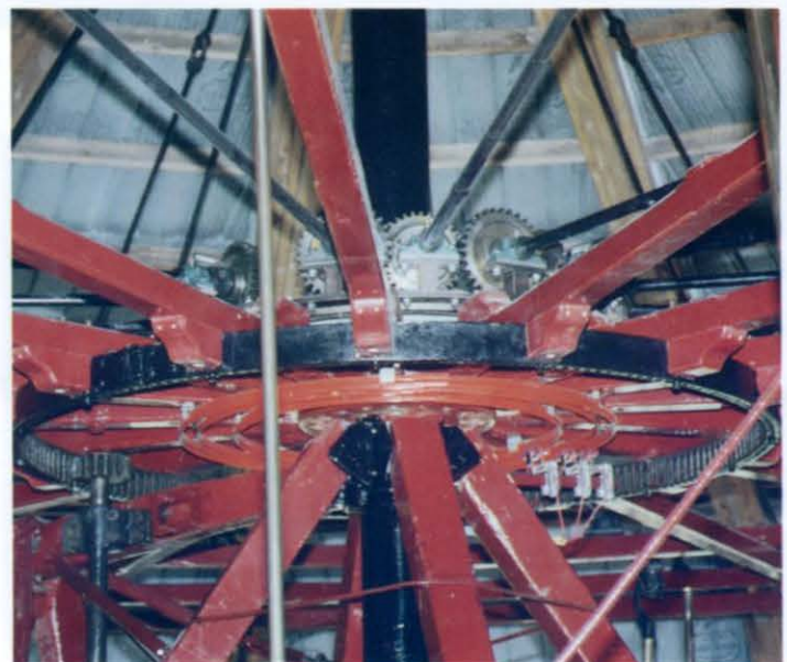
New gears replace the rubber tire drive system that was put on the carousel back in the 1970's.
