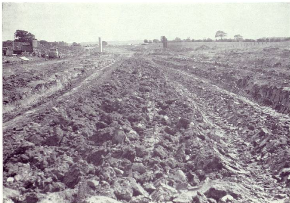
PLATE 3. Drainage (p. 62) General view of partially formed rig prepared by Caterpillar No. 16 Motor Grader.
