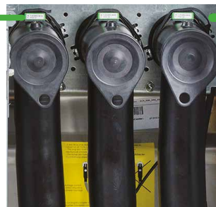
TH110 mounted on cable termination
