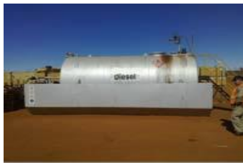
Bunded fuel storage
