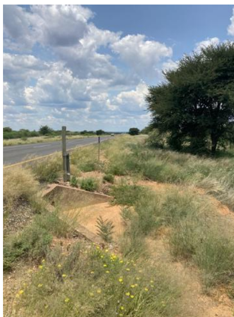
Figure 18 The pipeline will run along the R380 and cross through the above culvert to reach the extraction point on portion 1 of the farm Gloria 266
