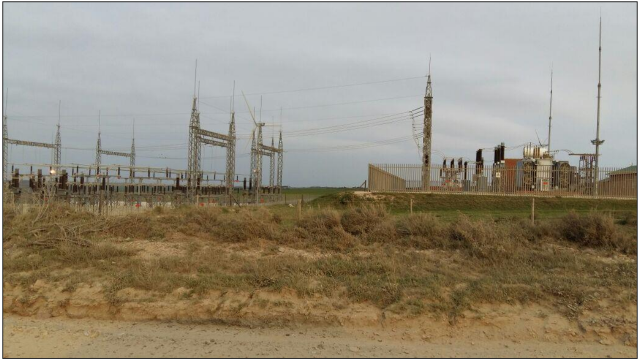
Figure 2-13: Example of a Wind Farm Substation (right) and adjoining Eskom Switching Station (left) on the Kouga Wind Farm
