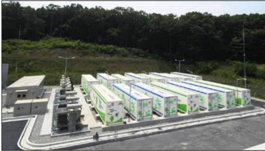
Figure 2-14: Example of a Lithium-Ion BESS installation
