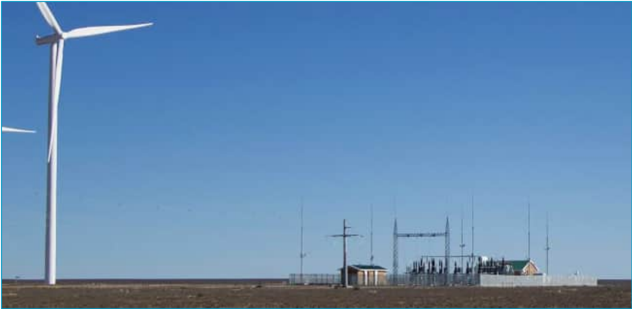
Figure 10: Example of typical substation associated with a wind farm
