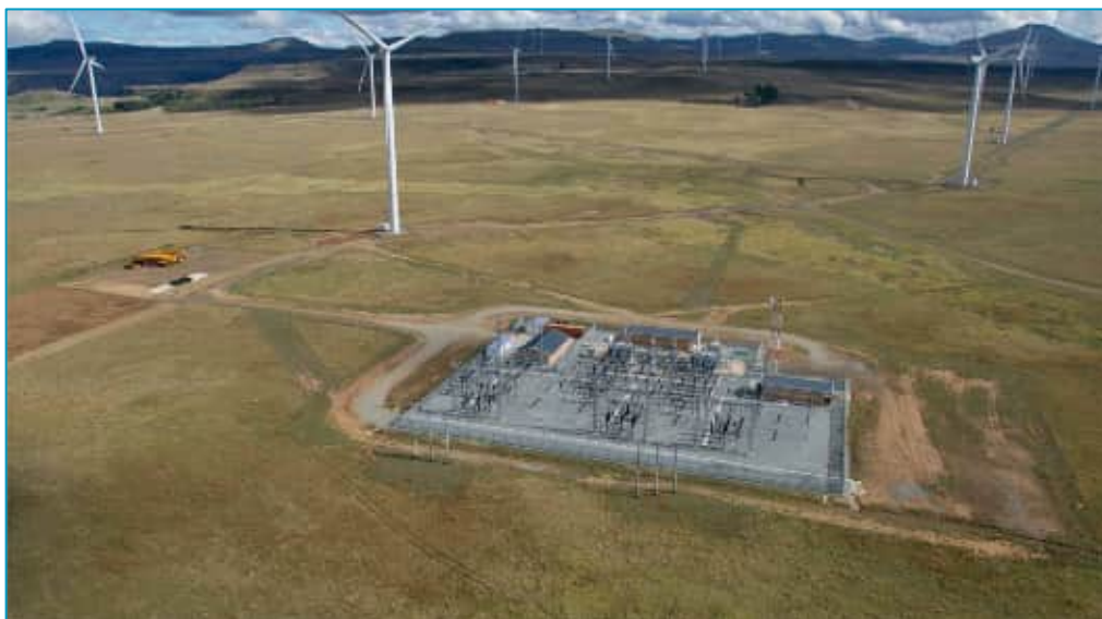
Figure 21: Example of a substation 7
