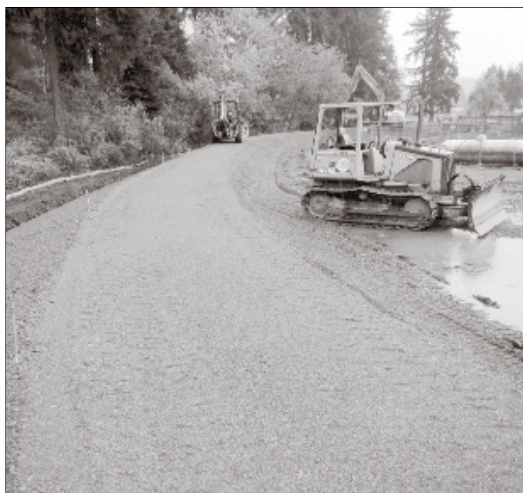
A bulldozer is seen at the site of a Bucoda levee, where improvements were recently made to protect the town's drinking water.
