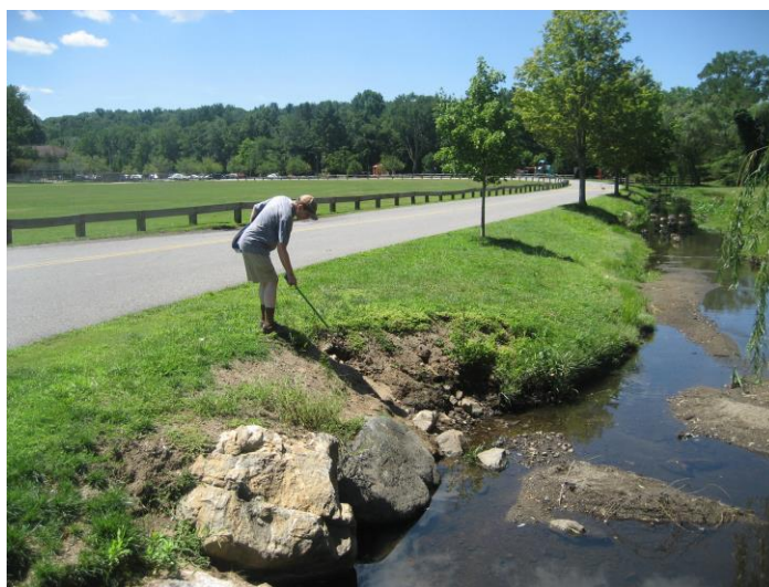
Erosion on eastern side of outlet caused by storm water culvert on west side of outlet
