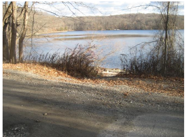
Asphalt/gravel interface at base of Byram Lake Road hill
