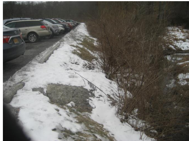
Runoff from MKMG parking lot
