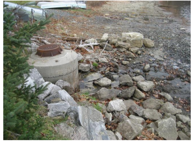
Water released into lake at pump station
