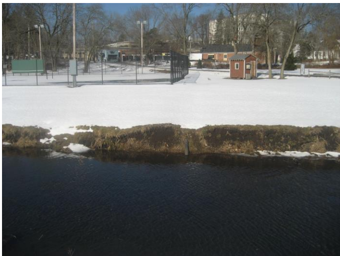
Looking west at unvegetated stream bank and erosion
