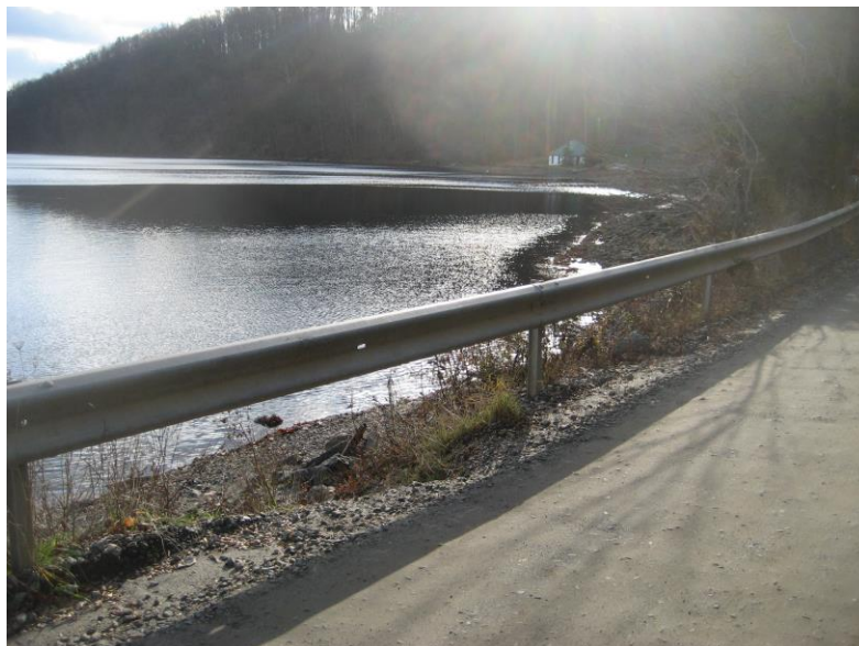
North end of lake from Byram Lake Road looking southwest. Lack of shoulders, curbing or vegetation allows storm water runoff directly into lake.
