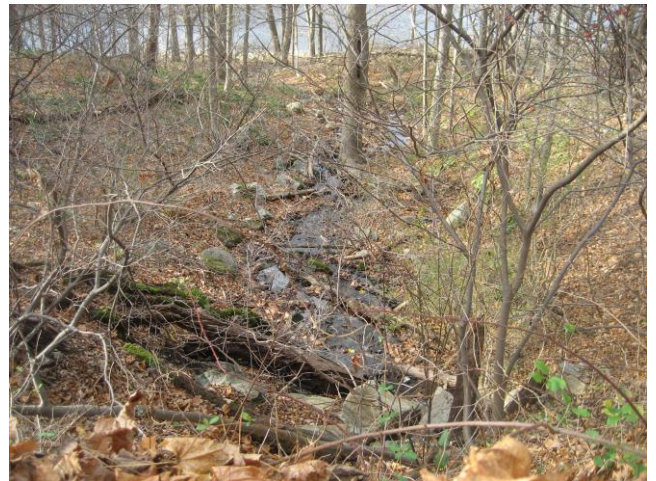
Collapsed headwall at BLT 6, looking west from road to lake
