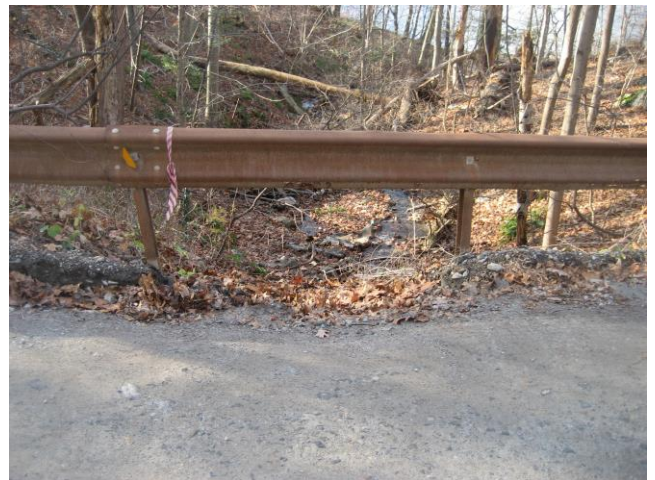
Looking west at road cave in at BLT 7
