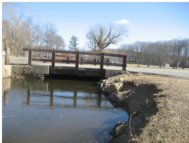
Looking north at unvegetated stream bank and erosion
