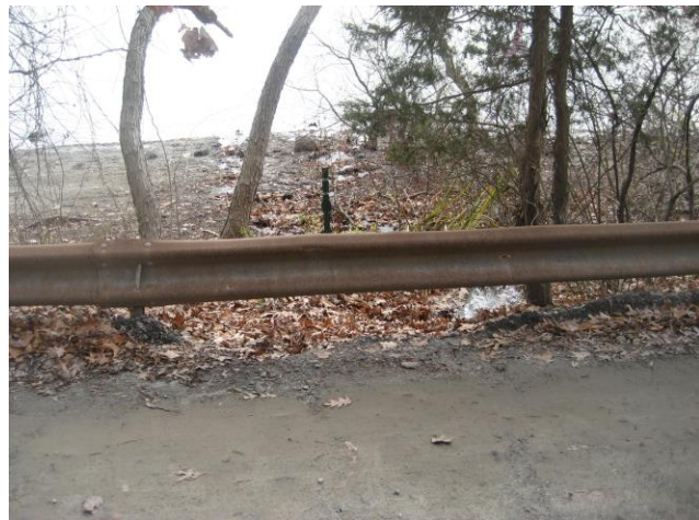
BLT 10 with no road shoulder or curbing
