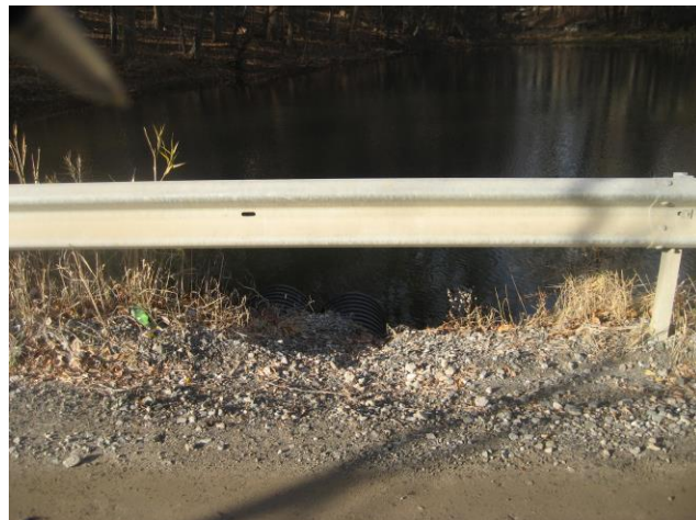
North side of Byram Lake Road is caving into the marsh
