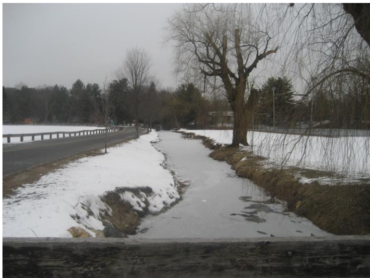
Wallace Pond outlet looking south, stream banks do not have vegetation to prevent erosion
