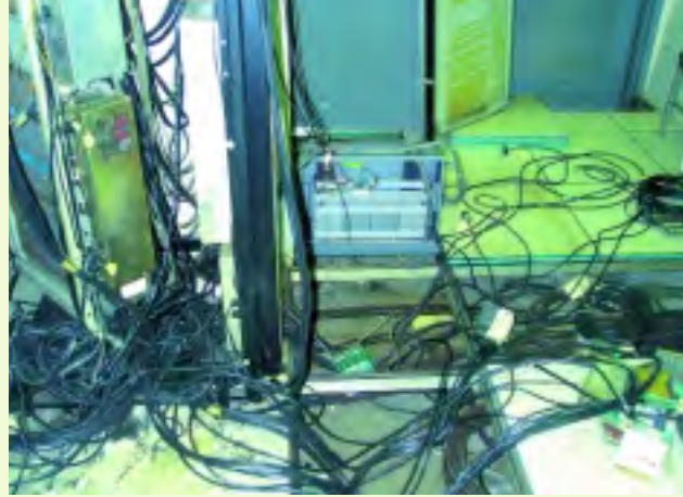
The weave of cables from cabinet to cabinet to power source were like a Gordian knot—almost impossible to untangle without a sword.
