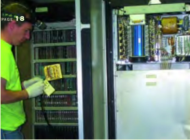
The cables were hard-wired into the cabinets and had circuit boards attached at various points.
