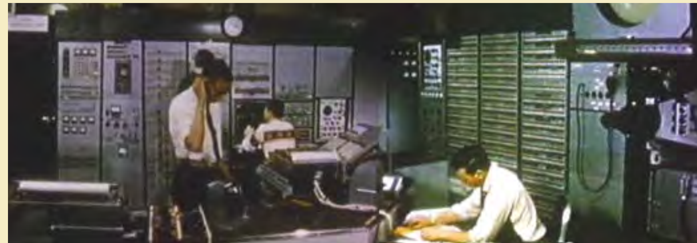
Whirlwind control room, 1954, from the film Making Electrons Count . Courtesy of MIT Museum.
