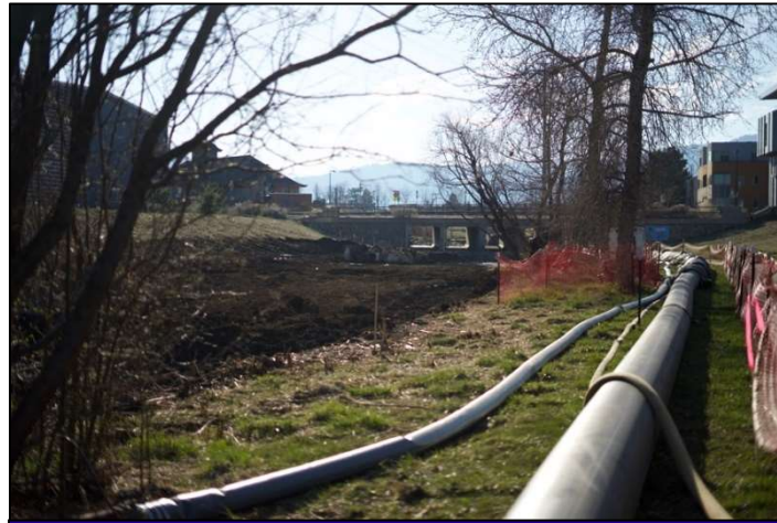
Modification of the Goose Creek Channel in preparation for seeding and planting. © Karissa Courtney
