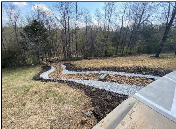
Bioswale accepting stormwater runoff at Mitchusson Park low-impact-development parking lot. © Eric Fuselier
