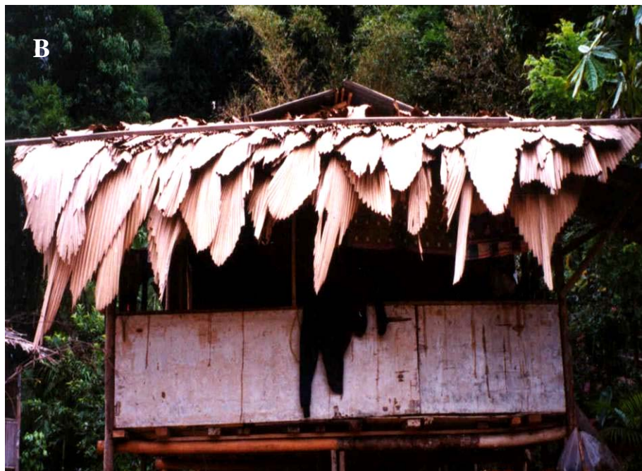
Figure 1.8.A. Roof made of leaves of Jt altifrons in the Endau-Rompin State Park, Johor, Peninsular Malaysia. B. The house of an aborigine family in Sungai Lalang, Hulu Langat, Selangor, Peninsular Malaysia, thatched with the leaves of Jt. magnifica .
