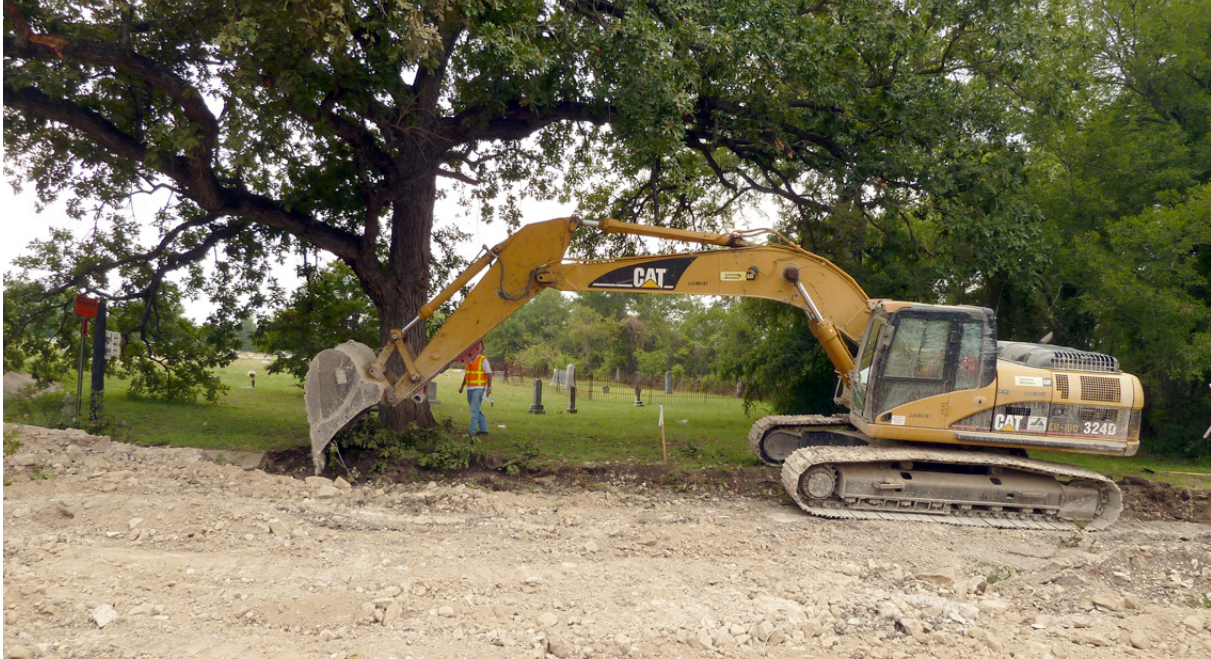
Figure 2.2. Initial stages of scraping using a trackhoe, looking west toward the cemetery.
