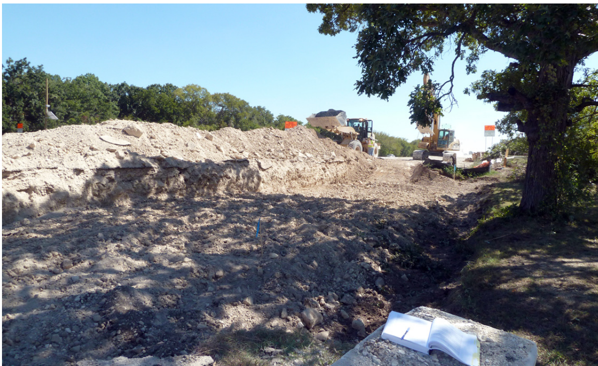
Figure 2.8. Stripping of the artificial fill from under the frontage road, looking south.
