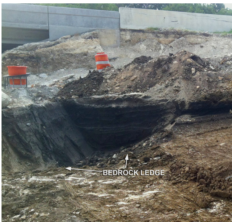
Figure 2.9. View eastward of the north end of the stripped area during early phases of systematic stripping. The far northern end has been stripped to bedrock, exposing a bedrock ledge and a deep pocket of dark clay in the northeast corner.
