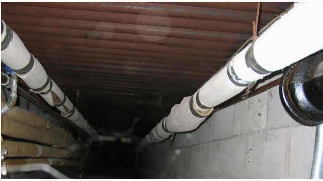
Asbestos pipe insulation prior to abatement in Oct. 2010
