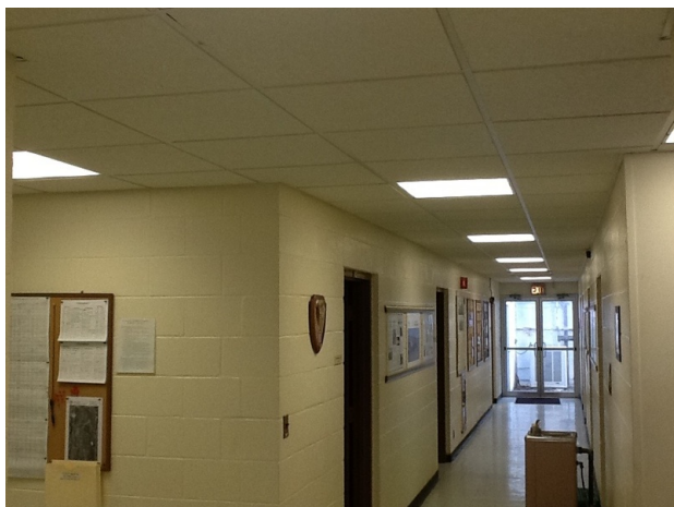
Rear hallway in HVRL building with new ceiling, and LED light fixtures
