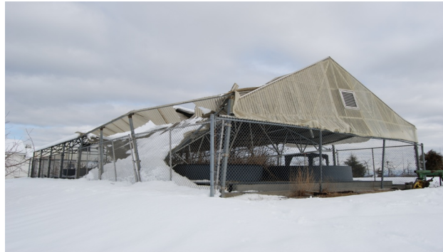
Collapsed roof of C.S.L.E.D. pavilion in Feb. 2010
