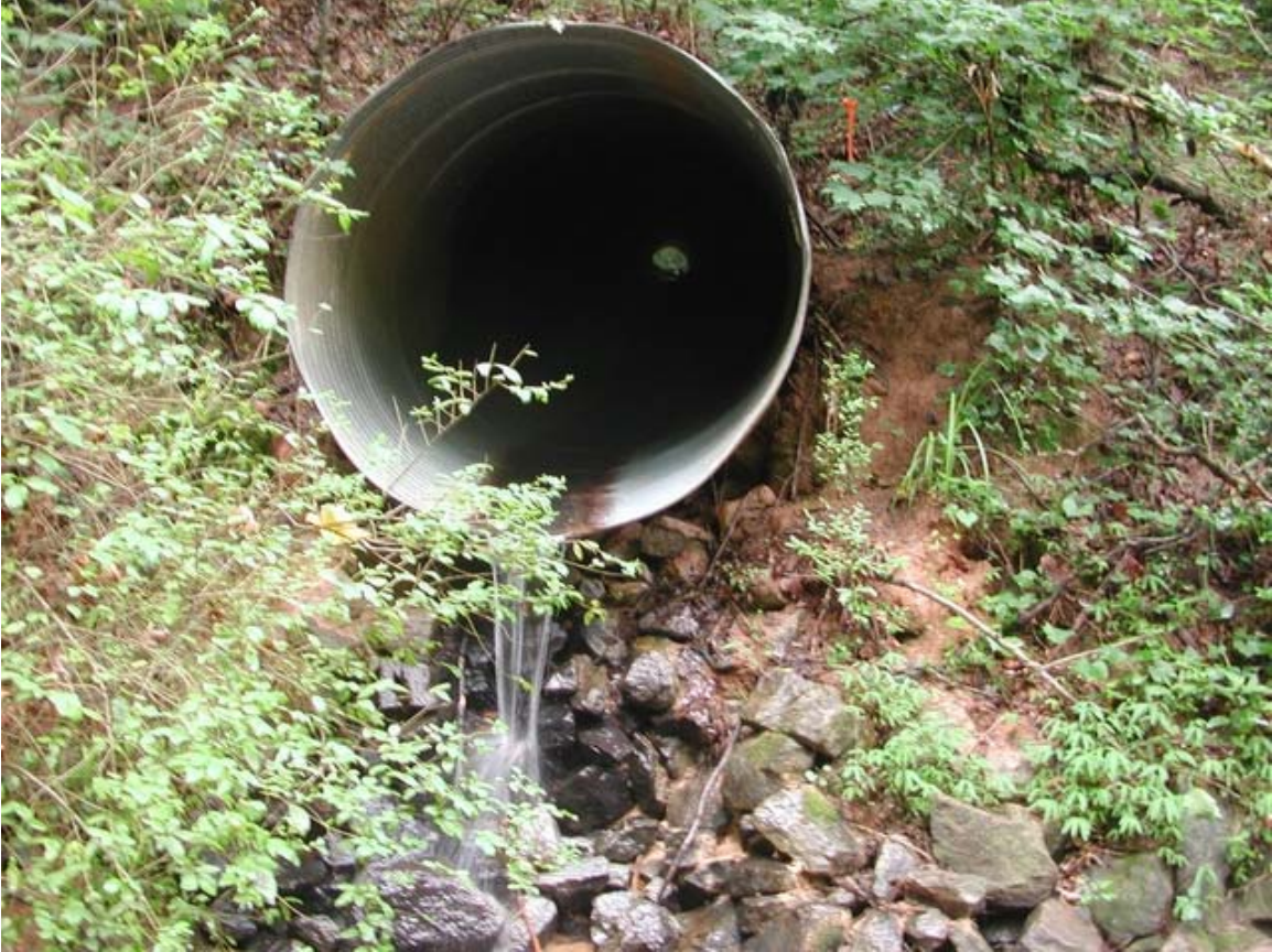
Figure 9: Stormwater outfall. Photo credit: Jeremy Pike.
