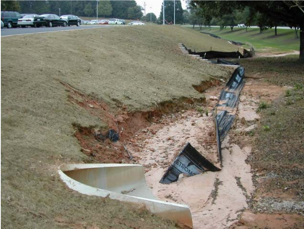
Figure 5: Eroded channel from uncontrolled stormwater
